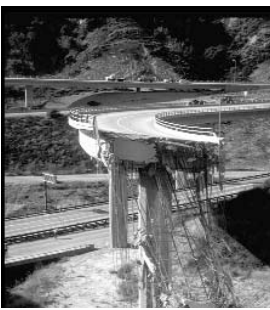
Figure 29-5 Damage from Northridge Earthquake, 1994
